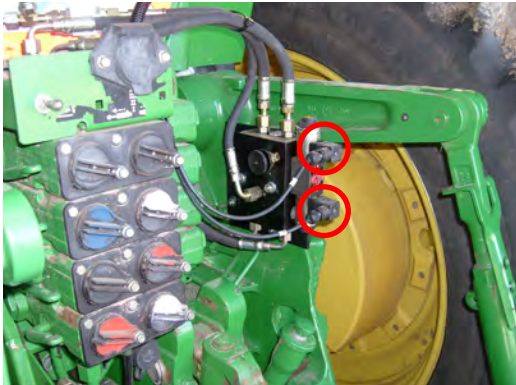
Figure 1-15: Control Cable Location
